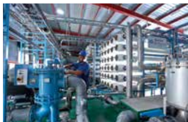
A seawater desalination system
