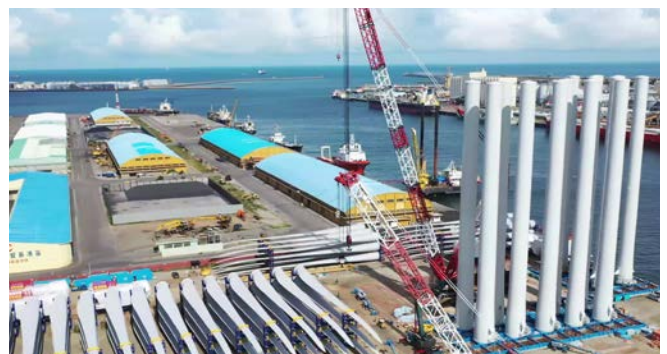
Pre-assembly work conducted at the Port of Taichung in the Changhua Offshore Wind Farm Project
