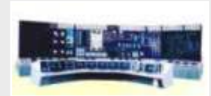
Main Control Room Panel
