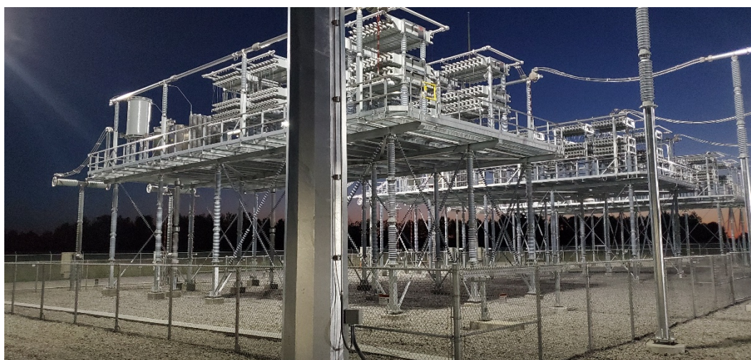
Warroad River Series Capacitor Bank
