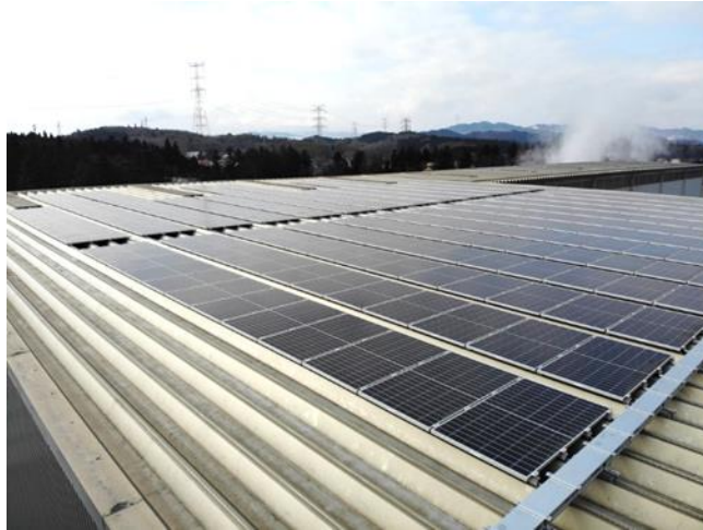
Solar panels installed on the roof of Hitachi Astemo High Cast's Fukushima plant
