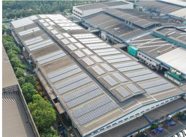
Solar panels on the roof of Hitachi Astemo Bekasi Manufacturing
