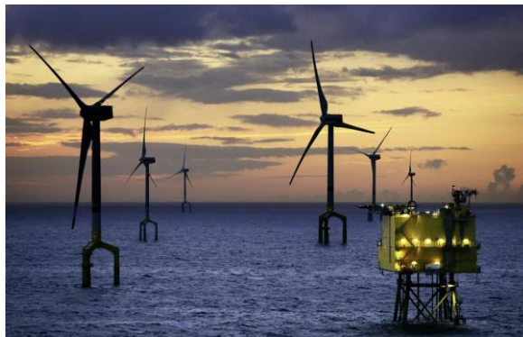
The first ever HVDC grid connection from an offshore wind farm, BorWin1 converter station in the North Sea
