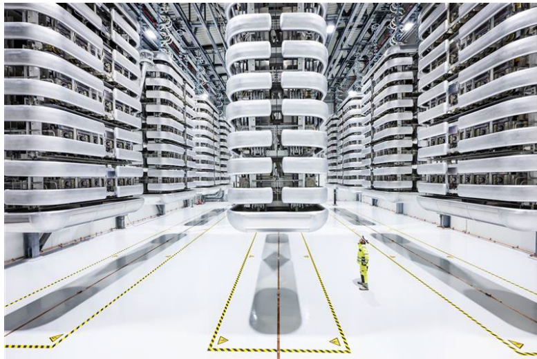
HVDC Light® Valve Hall
