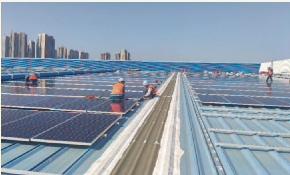
Figure 6 | Photovoltaic Panels at Escalator Factory
