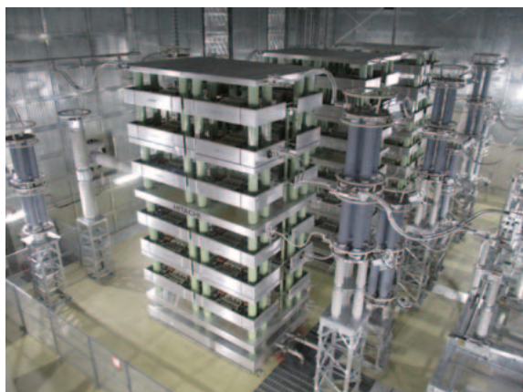
1 Hida converter station thyristor valves
