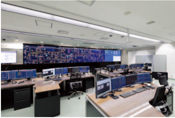
4 Kyushu Electric Power Transmission and Distribution System Electric Supply Control Station System
