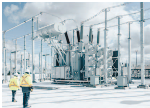
11 Achieve wide range of transformer maintenance
