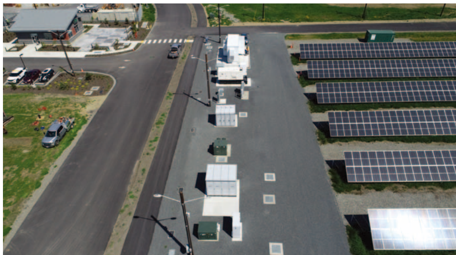
26 SnoPUD's microgrid and solar array
