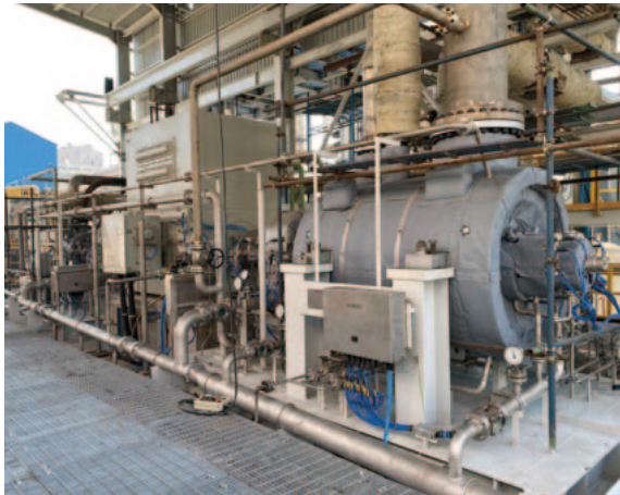
1 7,760 kW electric-motor driven CO 2 compressor (rear left: high pressure compressor, center: electric motor, front right: low pressure compressor)
