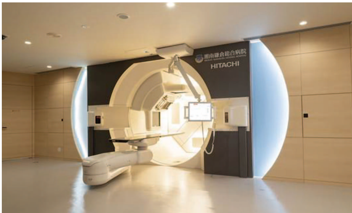
6 Proton therapy system treatment room in the Shonan Kamakura Advanced Medical Care Center
