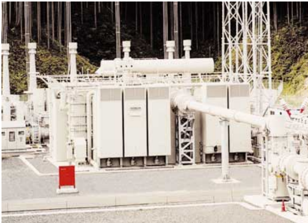
Fig. 4—500-kV 1,000-MVA Site-assembled Transformer for the Chizu Substation of the Chugoku Electric Power Co., Inc. The first-ever on-site assembly of a 500-kV transformer for Hitachi.
