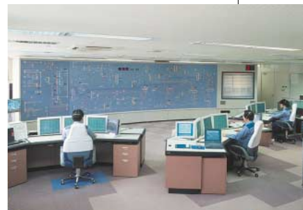
New LDC system, installed at the Osaka-Kita area load dispatching center, Kansai Electric Power Co., Inc.
