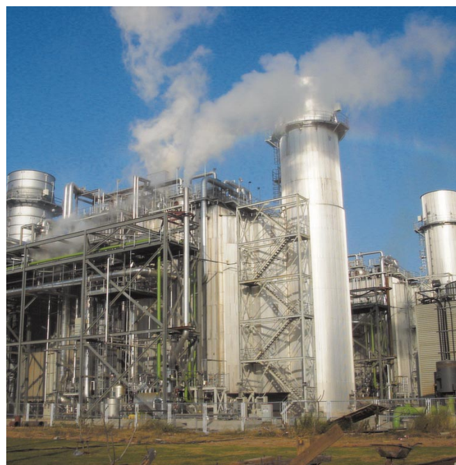
Overview of heat recovery steam generator for Ratchaburi Combined-cycle Power Plant Block-1
