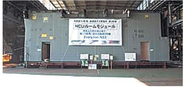
Fig. 8—HCU Module Assembly (5). Panoramic view of HCU room module is shown. This is the final phase before shipping (January 2008).
