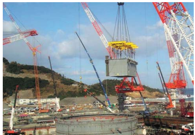
Fig. 9—HCU Module Installation. HCU was carried in by crawler crane at Shimane-3 site (February 2008).
