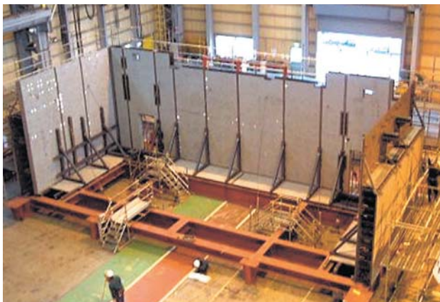
Fig. 4—HCU Module Assembly (1). SC (steel plate reinforced concrete) wall installation was performed by Kajima and Hitachi (January 2007).
