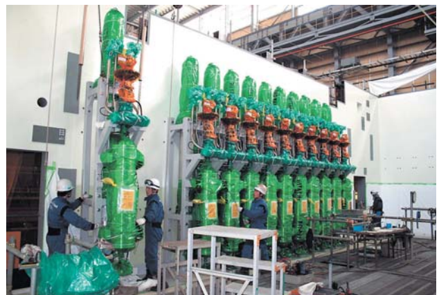
Fig. 5—HCU Module Assembly (2). HCUs were installed and anchor bolts were embedded on SC walls (March 2007).
