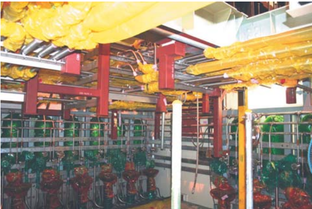
Fig. 7—HCU Module Assembly (4); Process Piping Installation. Installation of piping and support for the piping was completed (October 2007).
