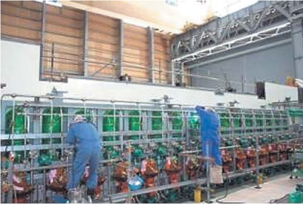
Fig. 6—HCU Module Assembly (3); Process Piping Welding. Process piping was welded and installed after HCU installation. This room module was shipped after all piping in the room was installed (May 2005).
