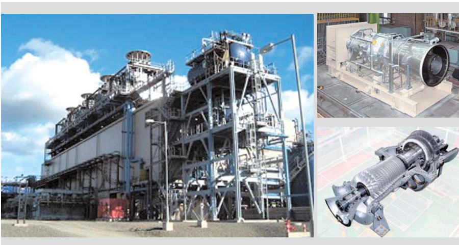
Fig. 1—H-25 Gas Turbine and General Overview of Sakhalin II Project in Russia.
