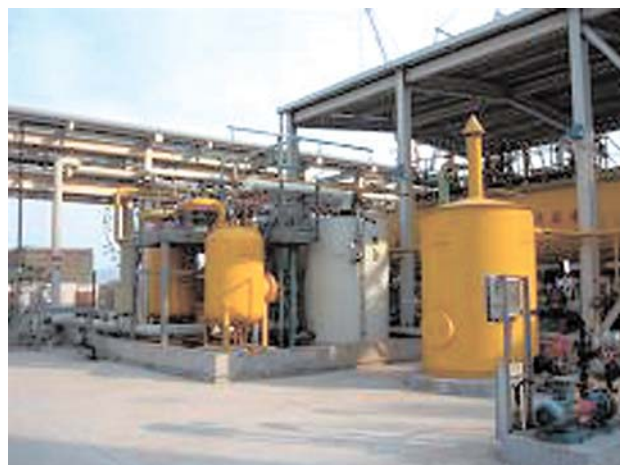
Fig. 4—External View of Ammonia Facility.
