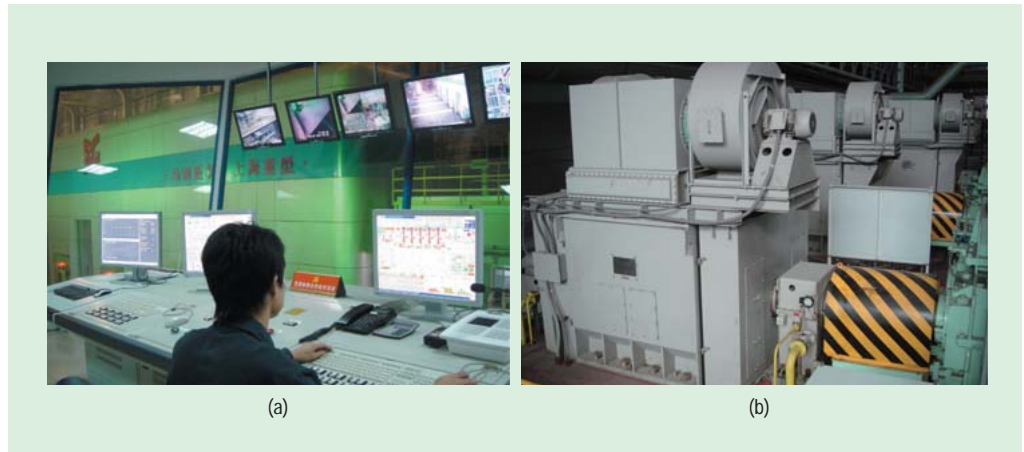
Operation room (a) showing one-person operation, and rolling mill main motors (b)
