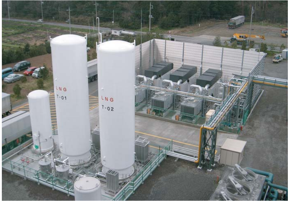
Appearance of ESCO facilities at Nihon Canpack Co., Ltd. Akagi Plant
