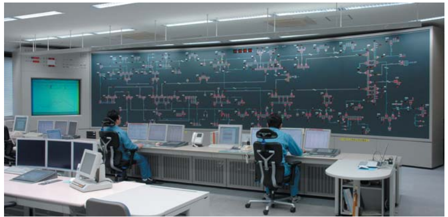
Aomori Regional Load Dispatching Center
