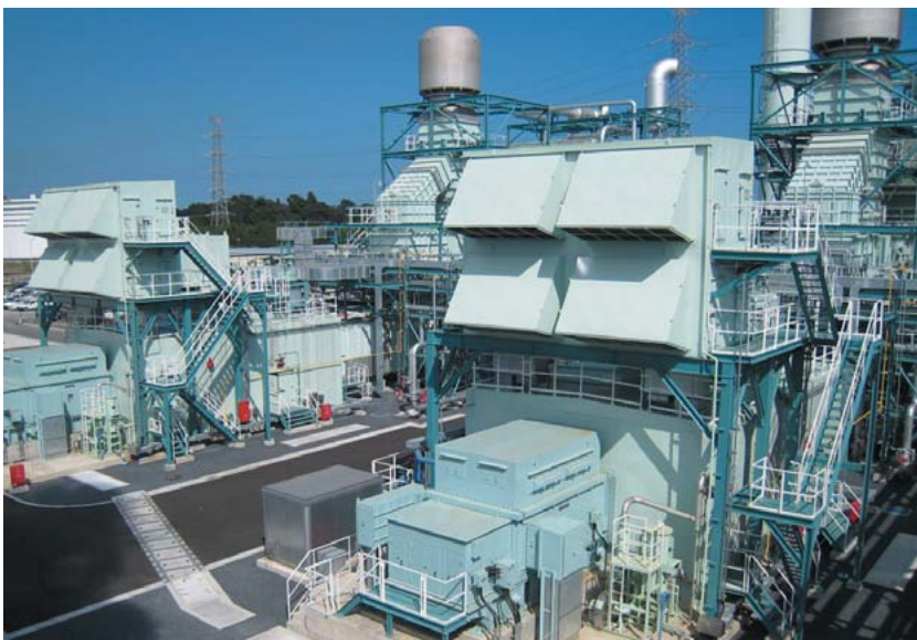
100-MW class high-efficiency H-25 gas turbine combined cycle power generation plants at Nippon Petroleum Refining Co., Ltd.'s Sendai Refinery
