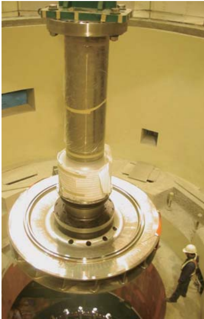
Installation of runner and shaft assembly of the No. 1 55.3-MW hydraulic turbine at Kukuan Power Plant, Taiwan Power Company
