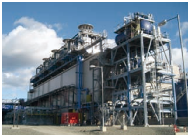
Fig. 8—H-25 Gas Turbine at Sakhalin II Project. An overview of the H-25 gas turbine that contributes to stable supply of LNG (liquefied natural gas).
