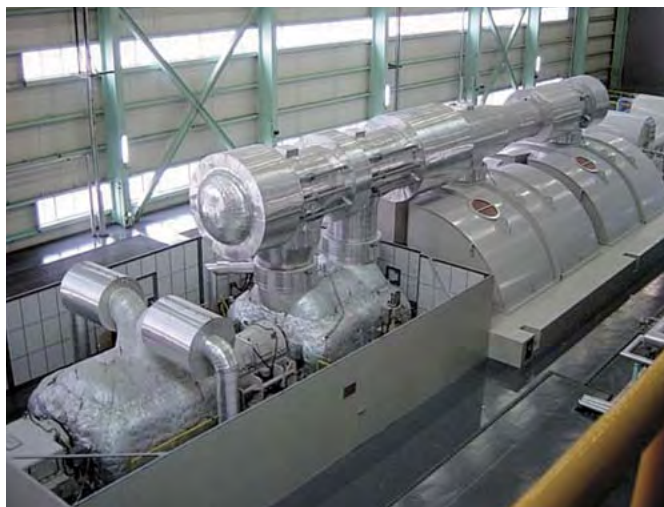
Steam turbine generator at Yeongheung Thermal Power Plant of Korea South-east Power Co., Ltd.
