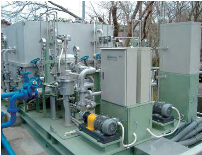
Ozone micro-bubble wastewater reuse system (daily capacity: 600 m 3 )
