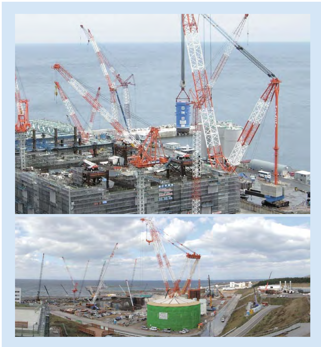
Reactor pressure vessel being carried into position by a large crawler crane at Unit 3 of the Shimane Nuclear Power Plant (top) and reactor containment vessel (front-center) being assembled at Ohma Nuclear Power Station (bottom)
