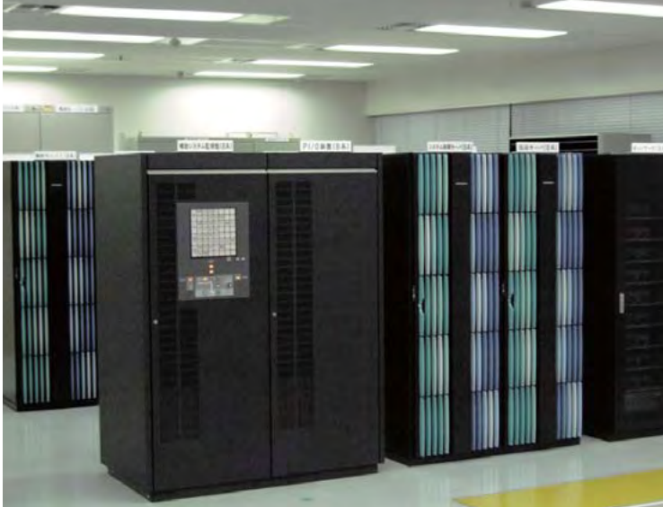
Online TSC system for Chubu Electric Power Co., Inc.
