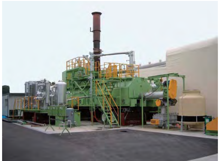
Indirect thermal desorption system
