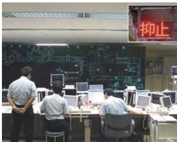
Large traffic display panel and stop sign display unit (top right) at Shin-Osaka General Control Center
