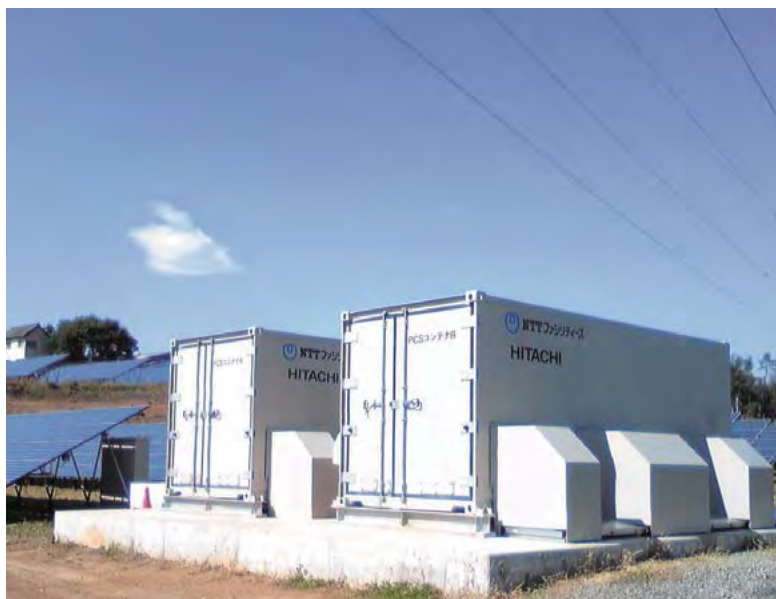
Outdoor cubicles for the 400-kW power conditioners installed at Hokuto
