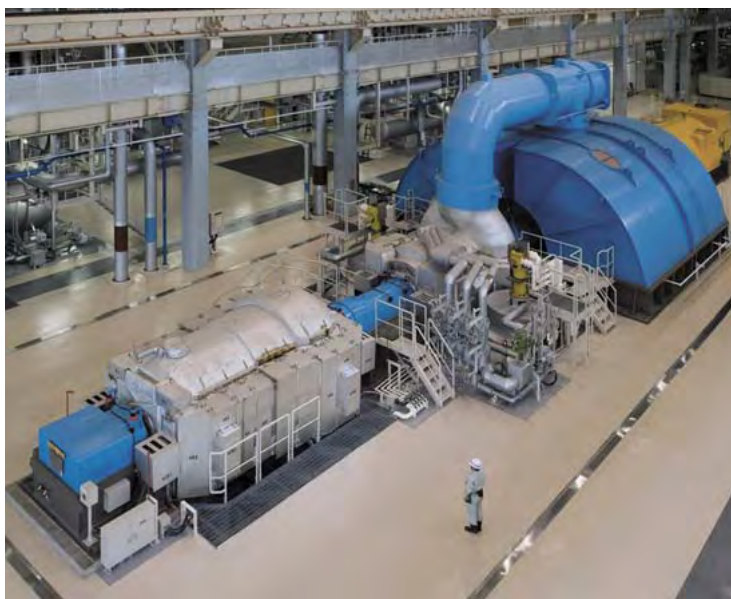
Steam turbine at Isogo Thermal Power Station of Electric Power Development Co., Ltd. (J-Power)
