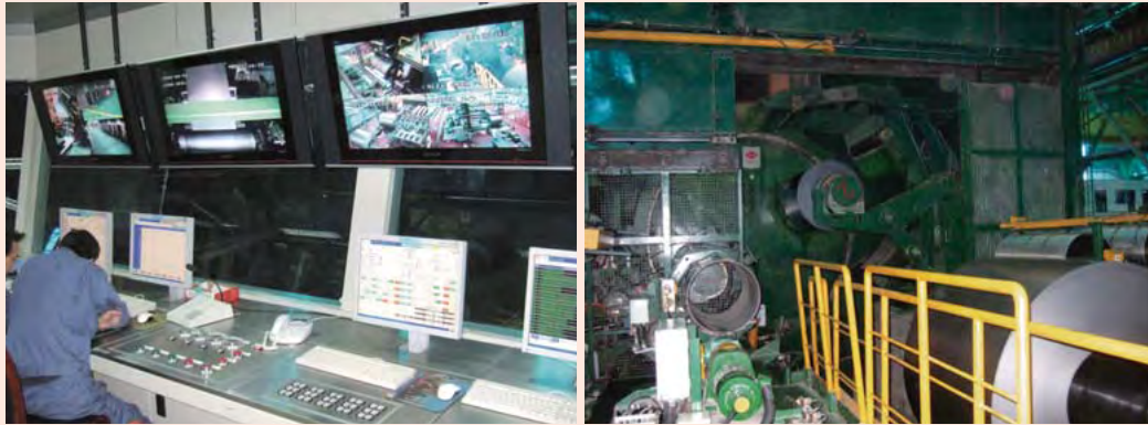
Control room (left) and tension reel (right) at wide continuous pickling line and cold rolling mill of Jiuquan Iron & Steel (Group) Co., Ltd.
