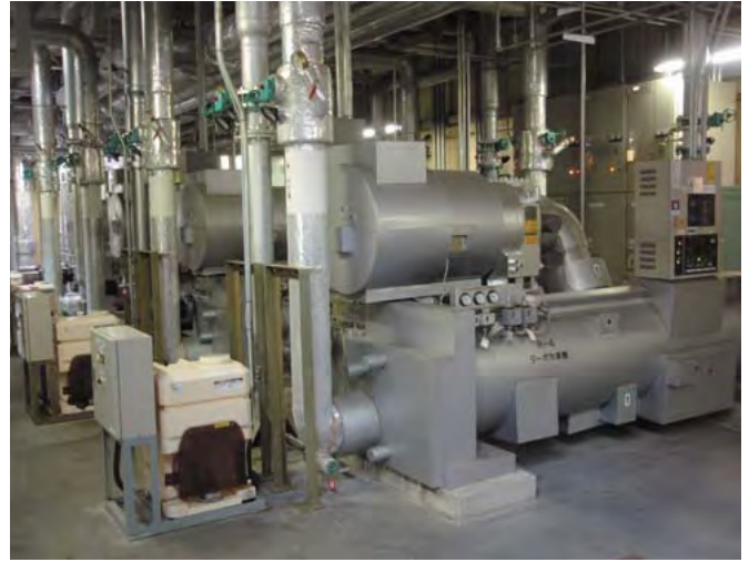
Turbo-cooler at Takasago Works of Hitachi Cable, Ltd.
