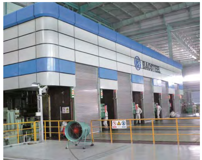
Electrical system for continuous pickling line and cold rolling mill for thin strip at Baosteel Group Shanghai Meishan Co., Ltd.
