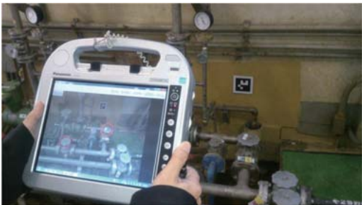
Use of augmented reality (AR) to provide instructions for equipment operation and maintenance work
