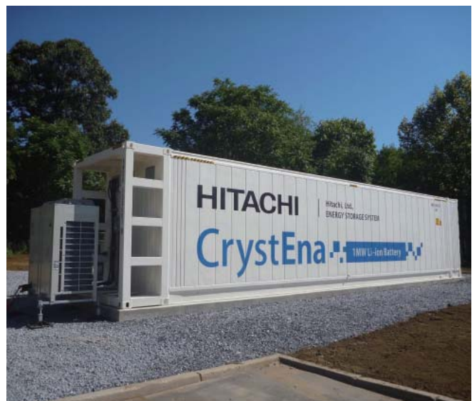
1-MW container-type energy storage system
