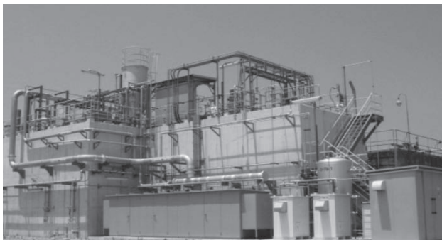
Fig. 7—Supplied Treatment System.
