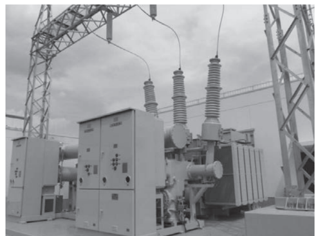
GIS: gas-insulated switch
