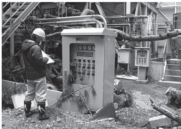
Fig. 2—Damage Survey in Progress. Conducting the survey on a site still bearing the scars of the disaster was a difficult task.
