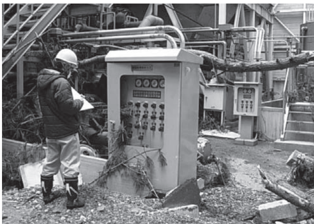
Fig. 2—Damage Survey in Progress. Conducting the survey on a site still bearing the scars of the disaster was a difficult task.
