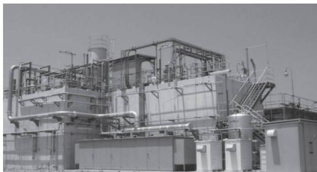
Fig. 7—Supplied Treatment System.
