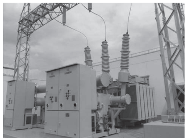
GIS: gas-insulated switch
