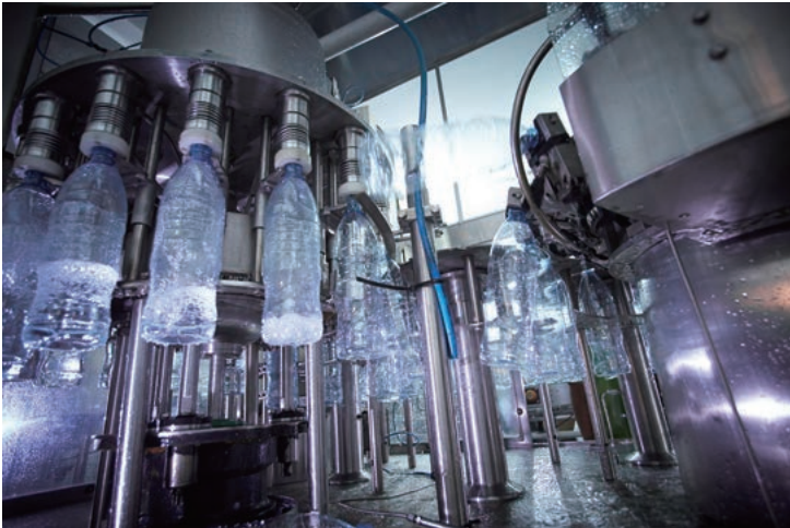
Seawater desalination plant (top) and drinking water bottling plant (bottom) in the Maldives
