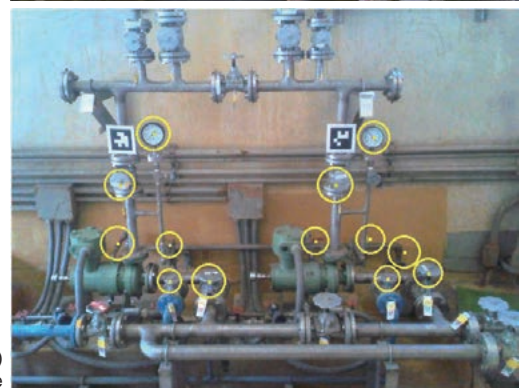
“Navigation system tool” that uses augmented reality (AR) to support operation and maintenance
