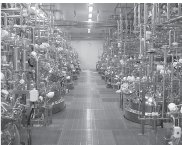
Fig. 1—High-volume Cell Culture System. This high-volume cell culture system (supplied by Hitachi, Ltd.) is used for the production of antibody drugs.
