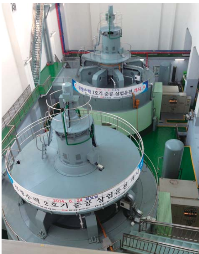
2 Cheongpyeong Hydro Power Plant Unit 1 (in the back) and Unit 2 (in the front) of Korea Hydro & Nuclear Power Co., Ltd. after completion of major overhaul
