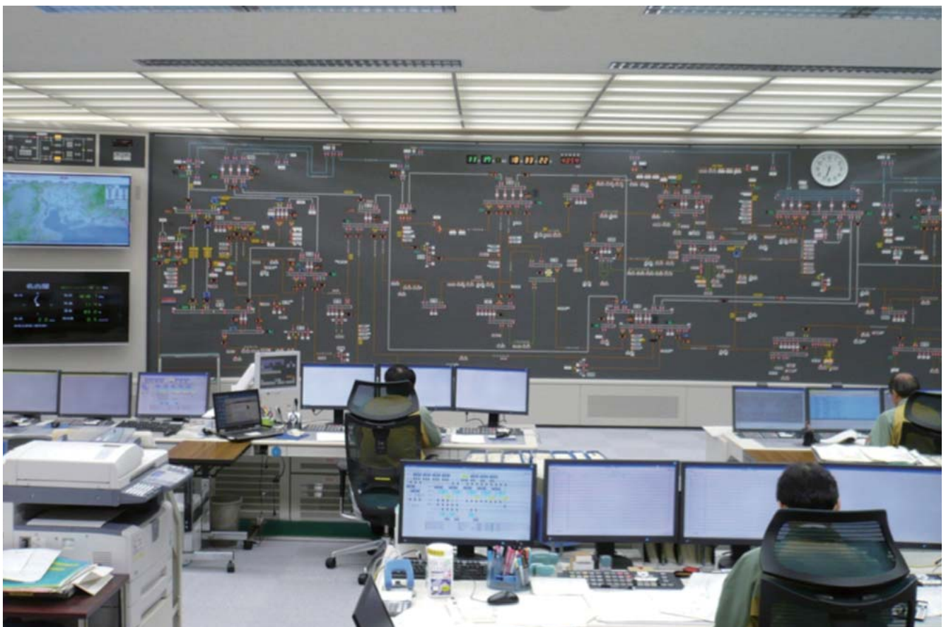
1 Meihoku Load Dispatch Control Center of Chubu Electric Power Co., Inc.
