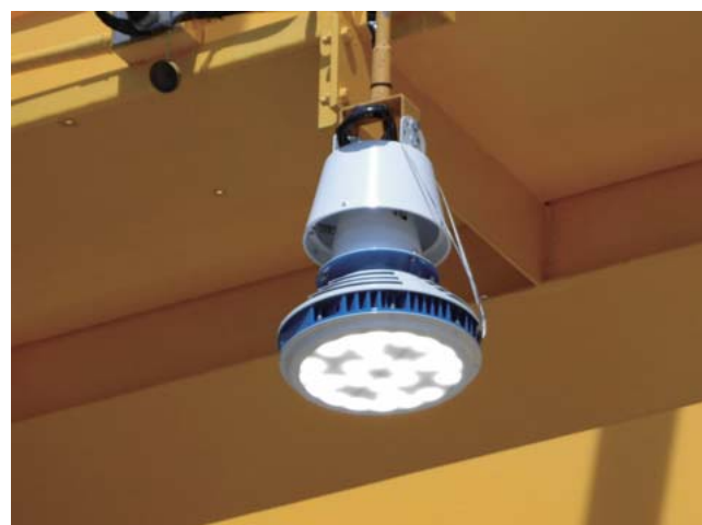
8 Industrial LED lights installed on a crane
