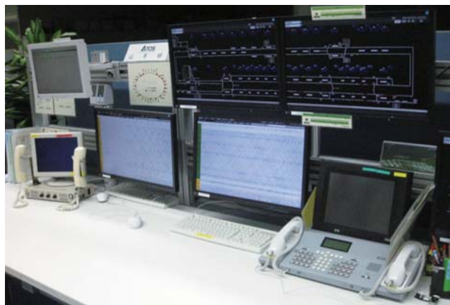
6 Control consoles of ATOS system for District 2 after upgrade
