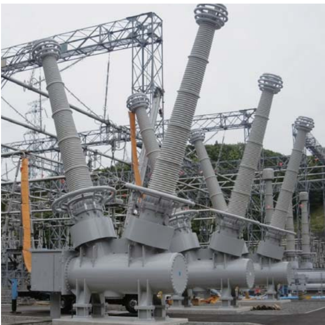
4 Installed 550-kV GCB
