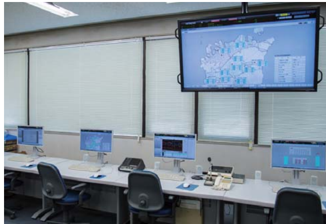
2 Central control room of monitoring and control system at the Water Supply Management Center of Niihama City Waterworks Bureau
