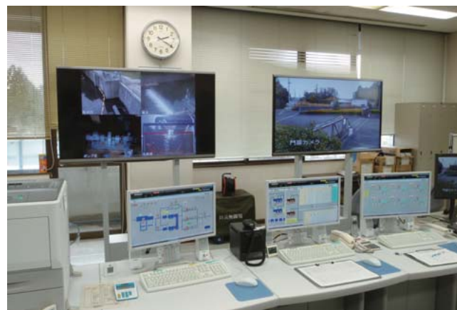
4 Central monitoring and control system for Hinumagawa River Water Purification Plant of the Ibaraki Prefectural Public Enterprise Bureau
