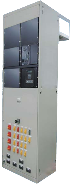
2 275-kV current differential protective relay panel
