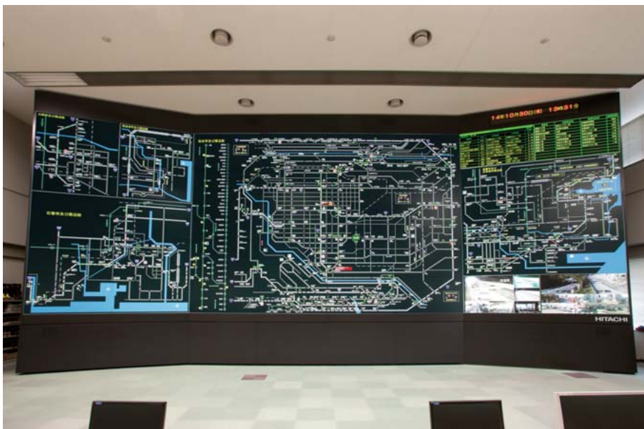
8 Traffic conditions display panel system for Miyagi Prefectural Police Headquarters
