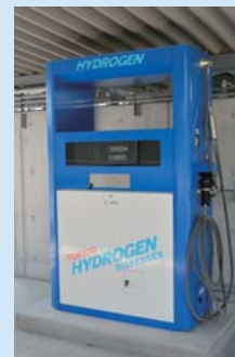
6 High-pressure, high-capacity compressor (top), accumulator (middle), and dispenser (bottom)
