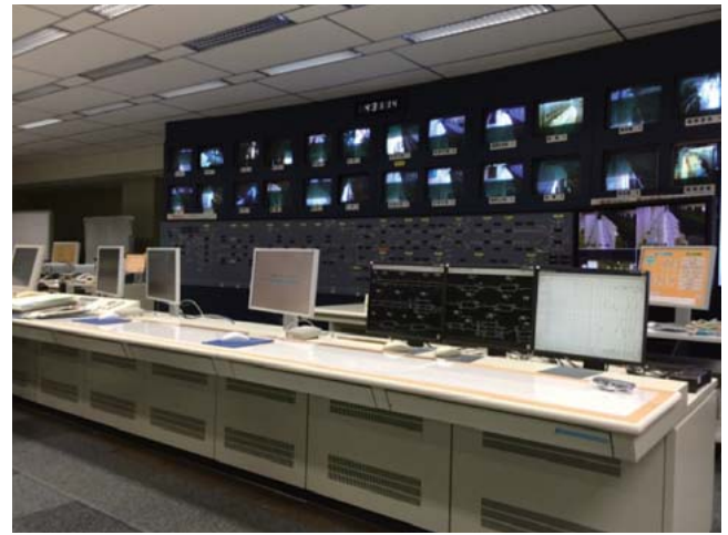
3 Traffic displays and control desks for traffic management system of Fukuoka City Subway
