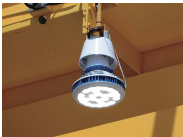
8 Industrial LED lights installed on a crane
