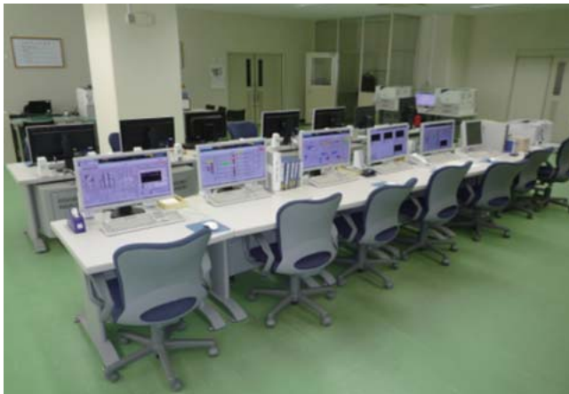
1 Monitoring and control system for Sorami Sludge Recycle Center of Nagoya City Waterworks & Sewerage Bureau
