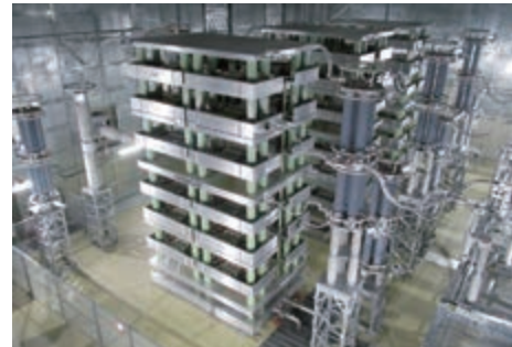
High-Voltage Direct Current (HVDC) AC/DC converter (Hida Converter Station of Chubu Electric Power Grid Co., Inc.)
