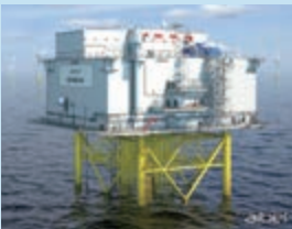
HVDC (high-voltage direct current) converter station
