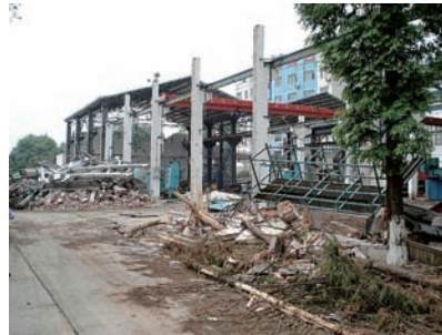
(Top) Hitachi Construction Machinery excavators, important for earthquake recovery (Bottom) Earthquake damage at Dongfang Electric Corporation's Hanwang plant
