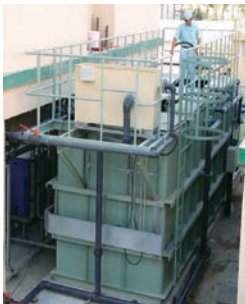
A PERSEUS system installed at a construction workers' housing complex in Dubai processes wastewater for about 1,500 people
