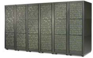
Enterprise storage platform
