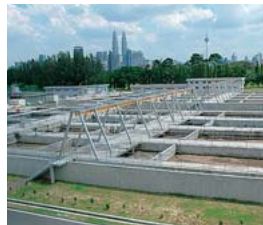
Bunus sewage treatment plant in Malaysia
