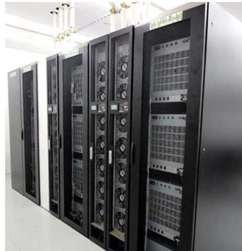
Modular data center
