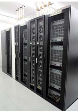
Modular data center
